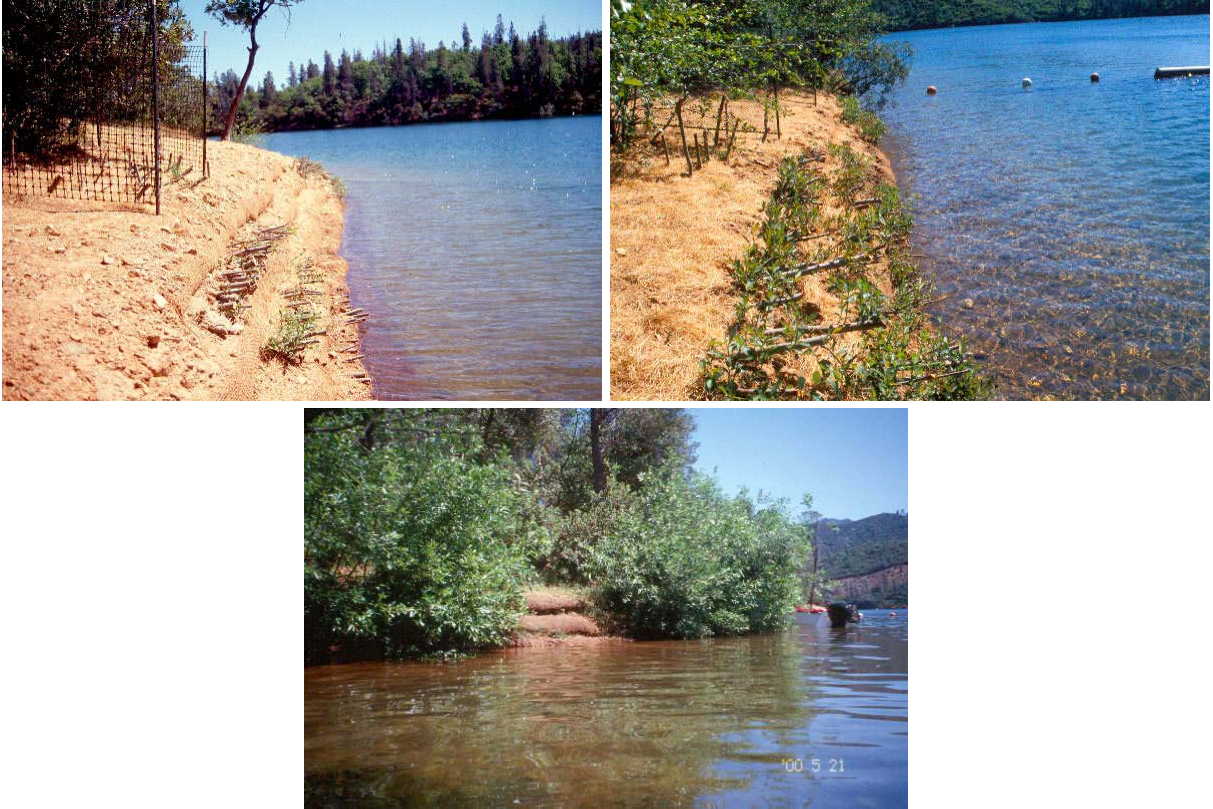
Brushlayering with soil wrap was used to stabilize and revegetate eroding banks at Whiskeytown Lake, Whiskeytown National Recreation Area, CA.
