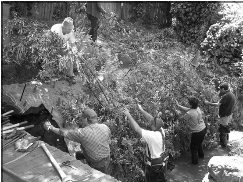
UCC staff lead a demonstration project on Codornices Creek in Berkeley. Local homeowners learned how to install soil bioengineering methods to prevent erosion, such as the brush mattress seen here.
