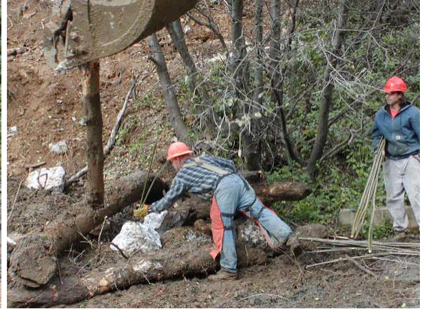
Workers place willow poles into the hole left by the oak "Stinger".
